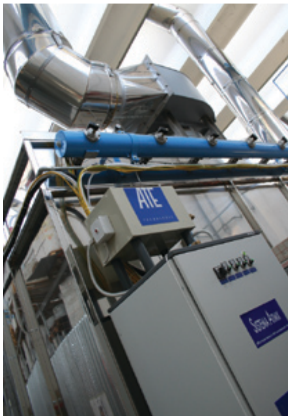
4 - The Atimix equipment installed in one of the two manual powder coating booths.
