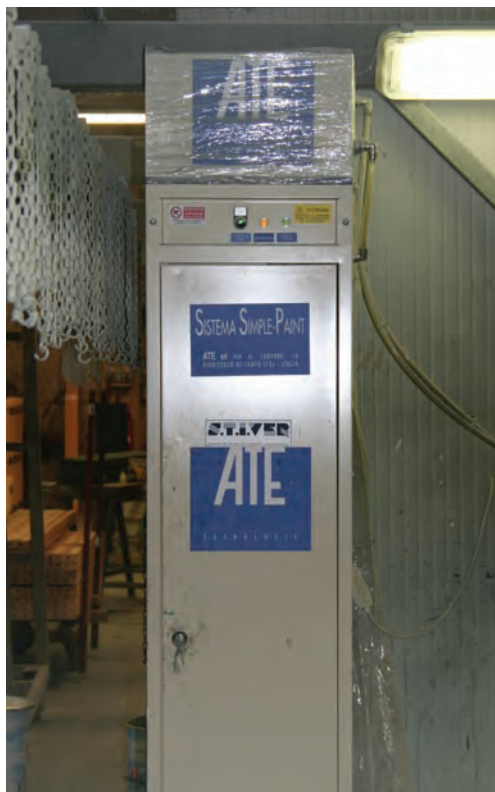
5 - The Simple Paint enhanced application system from Ate, installed by Stiver in the painting cabin.
